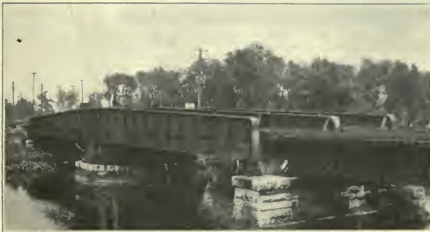
FIG. 271. BRIDGES. Plate-girder draw bridge of the Illinois Central Railroad over the Grand Calumet River at Riverdale.
